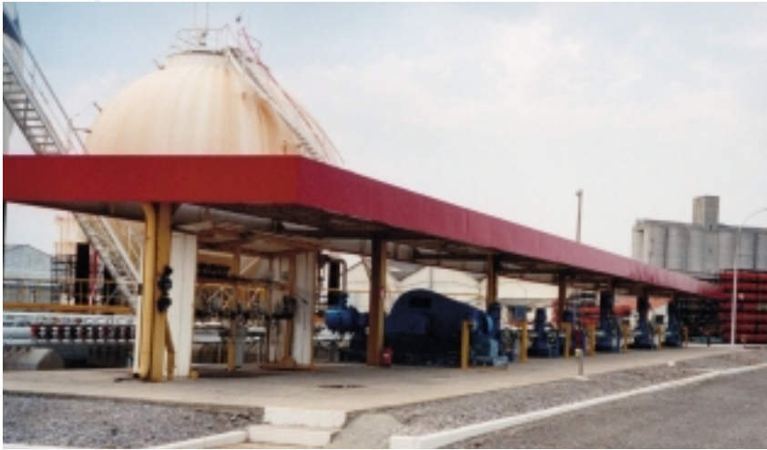
Quay of loading LPG
