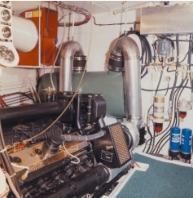
Example : Boiler room
